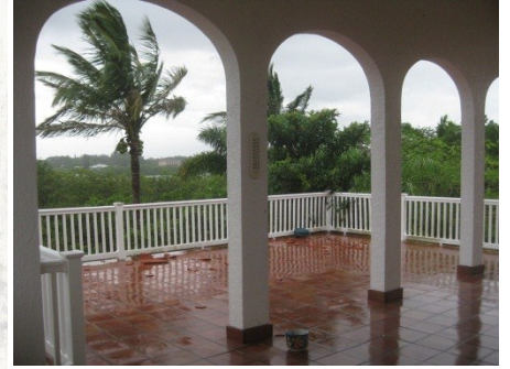
Even small hurricanes crash tiles
